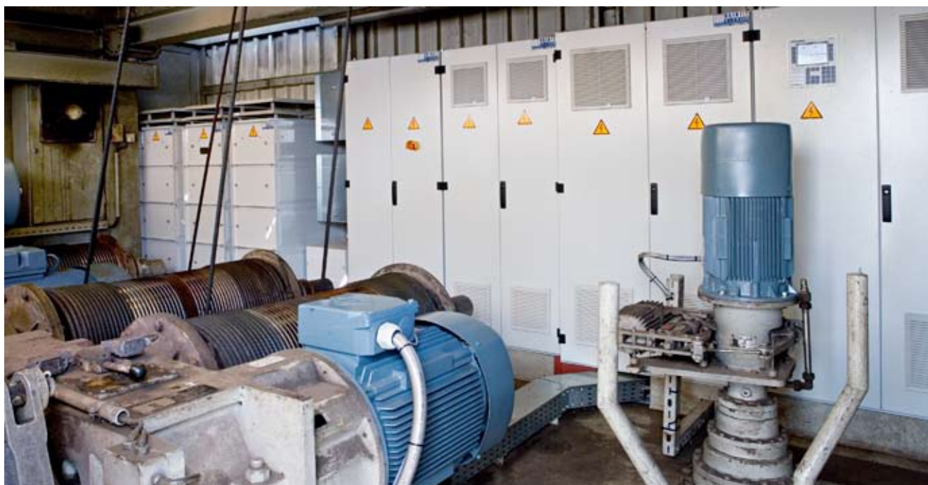
Emotron was responsible for engineering, delivery of the motors, construction of the cabinet equipment and commissioning.
