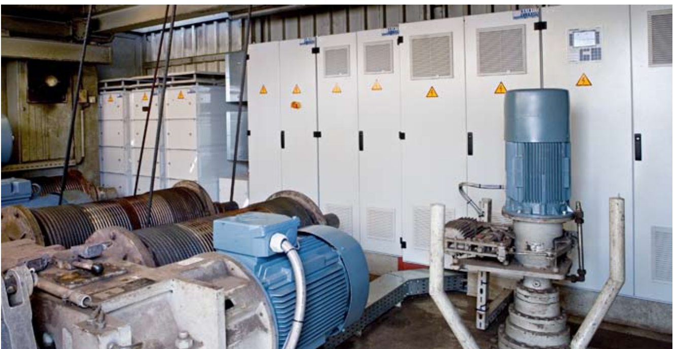
Emotron was responsible for engineering, delivery of the motors, construction of the cabinet equipment and commissioning.
