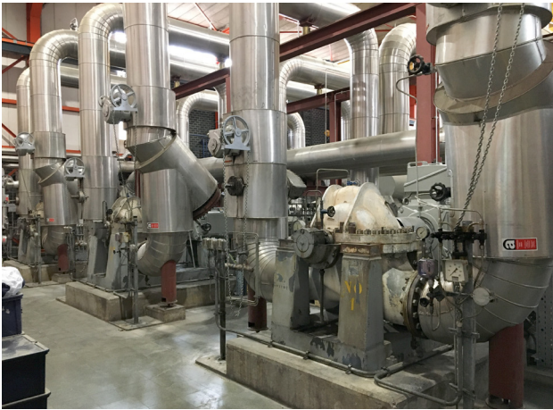
3 renovated pump lines with AC motors.
