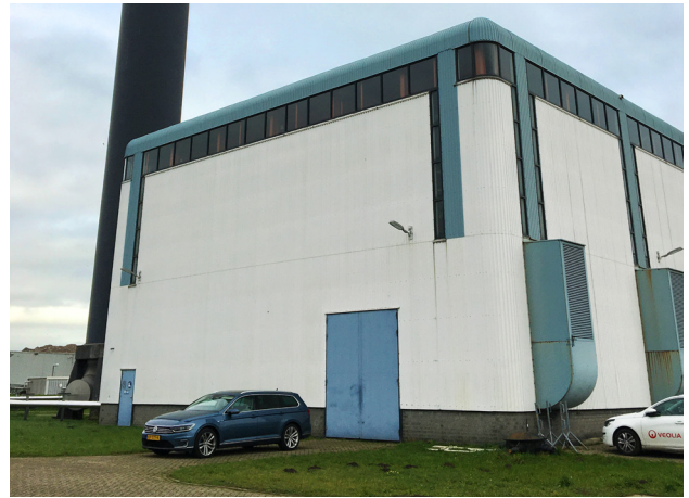
The pump station in Breda maintaining correct pressure and temperature.
