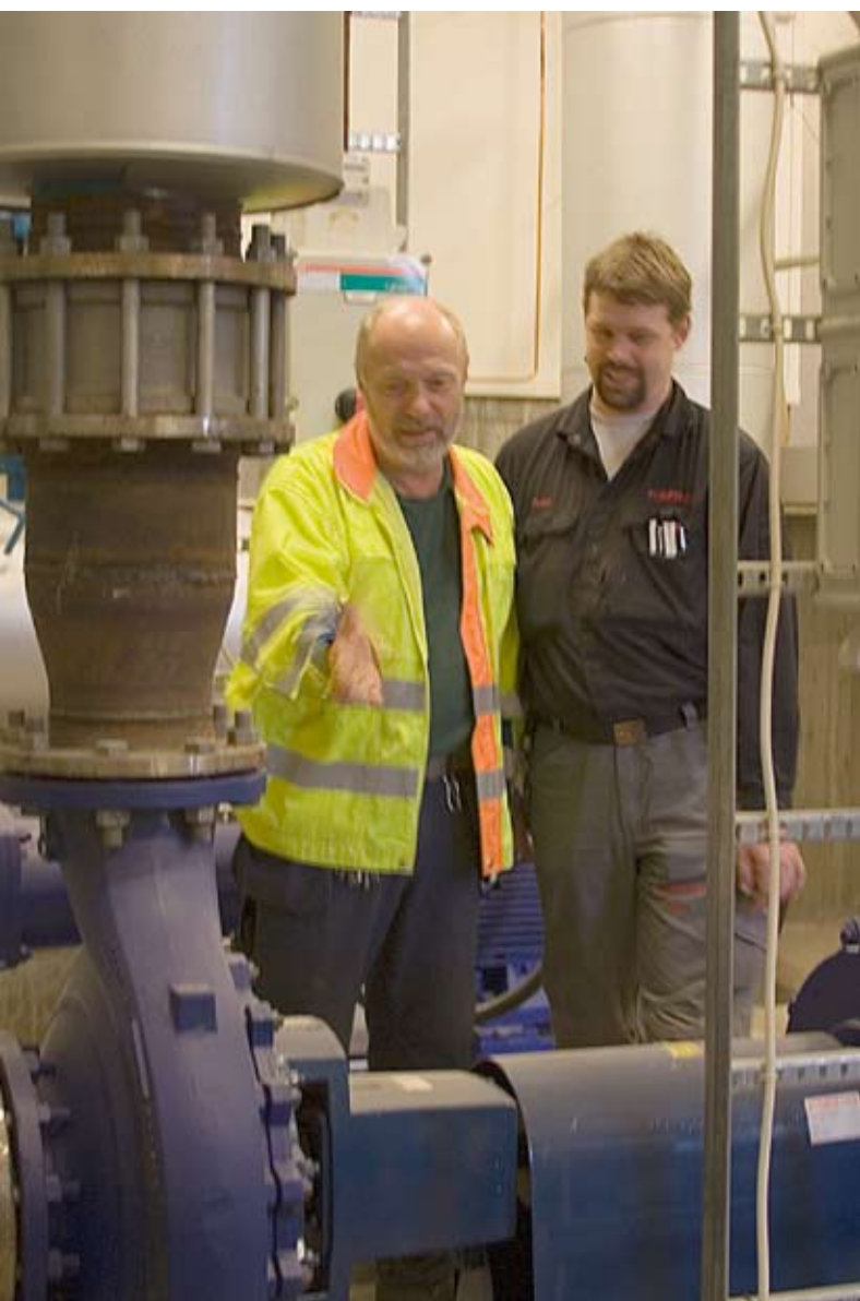
Three pumps maintain the pressure in the district heating network's pipes. Peter Johannisson (r) and Franc Rostedt (l) are very pleased with the extended functionality of the new Emotron FDU 2.0. “The built-in shaft power monitor prevents dry-running and we can control several pumps with just one variable speed drive,” says Peter.
