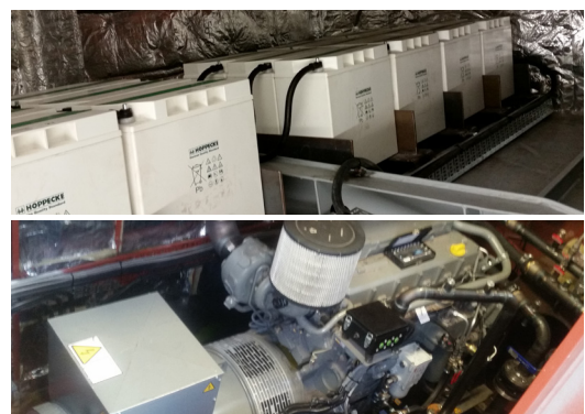
DC supply from a battery pack or generator AC supply.
