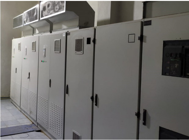
Cabinet build housing Emotron VFDs
