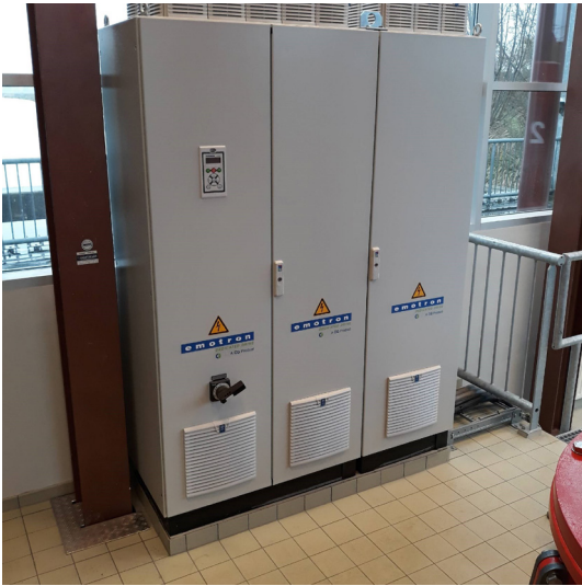
Emtotron VFXR 2.1 AFE in cabinet build
