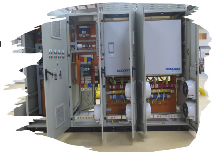
Emotron VFDs in cabinet
